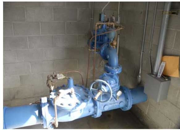
Well No. 3 - Valving
