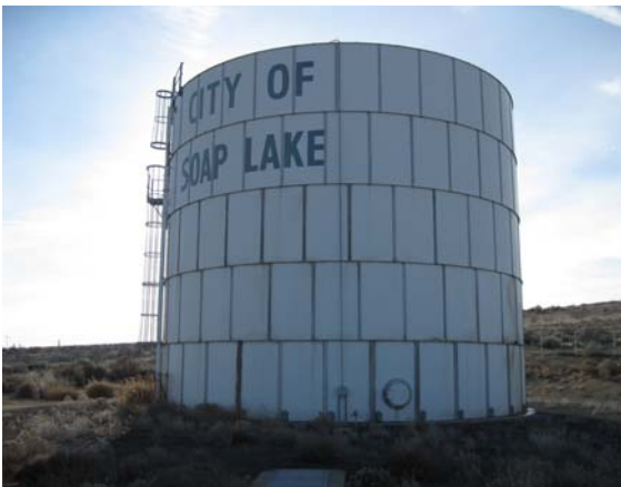
500,000 gal Bolted Steel West Reservoir
