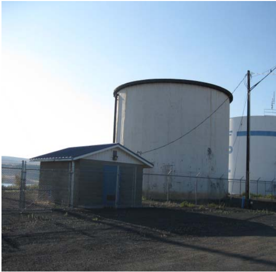
BPS, 300,000 gal Concrete Reservoir (not in use), East 500,000 Steel Reservoir
