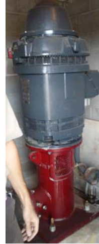
Well No. 1 – Motor and Piping
