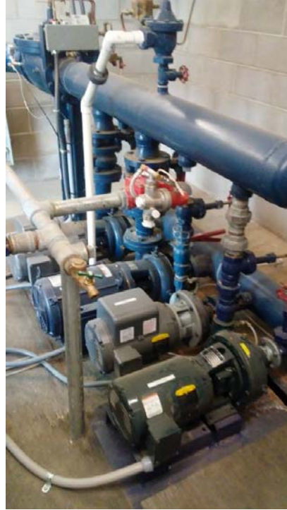
BPS Pumps and Piping
